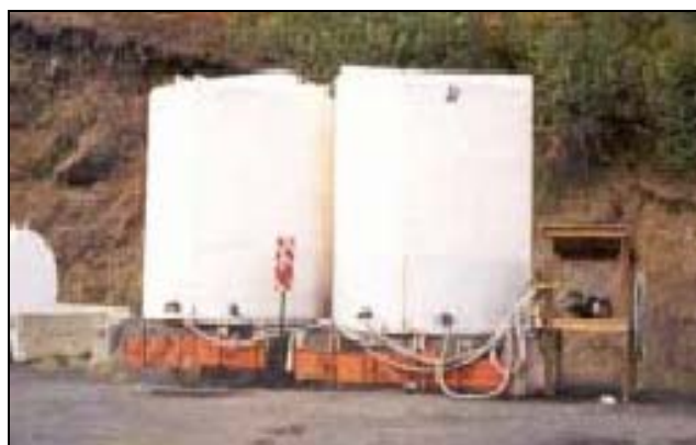
Idaho DOT Chemical Storage Tanks
